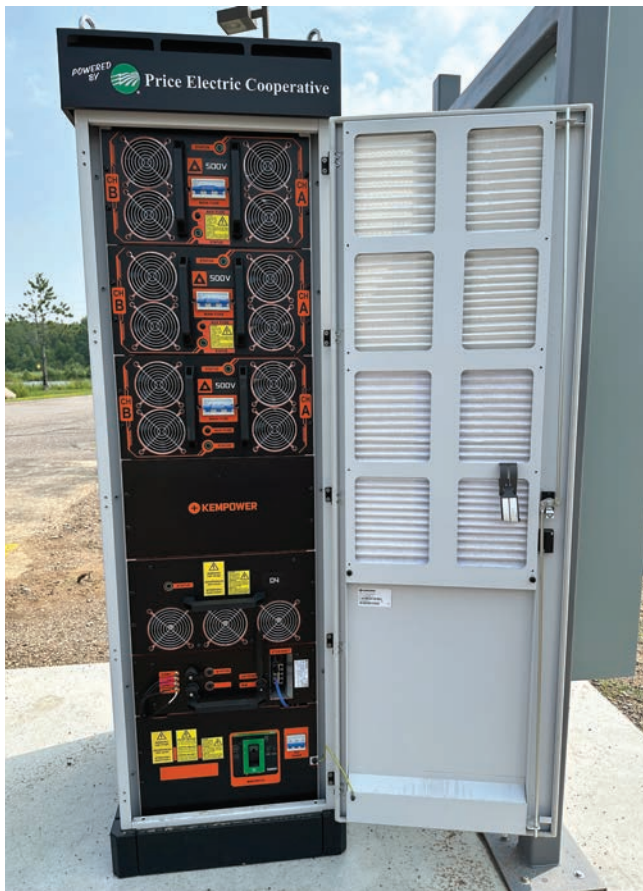
Shown above is the modular design of the EV charger. There is one open slot for an additional 50kW module.
