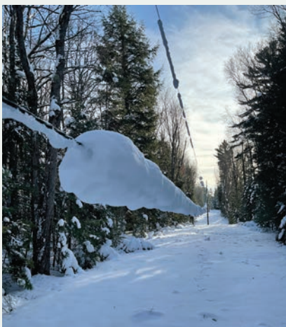
This power line is significantly weighed down due to snow load. This photo was taken in the Springstead area.
